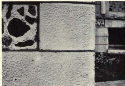
An Excellent and a Poor Example of Concrete Finish. The Corner Stones Are Finished With the Pointer and Appear Well. The other Stones Have Aggregate of Too Large Size Impressed Into Surface.
