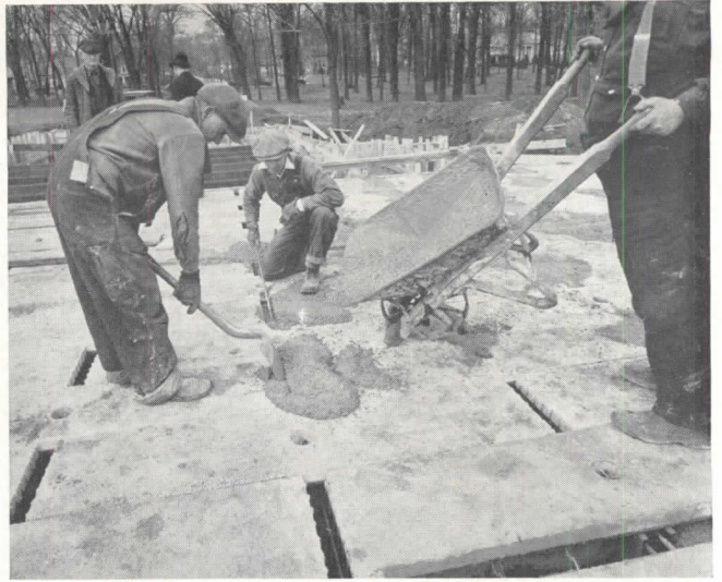
stagger arrangement (see diagram) on the steel forms; concrete beams are then poured (above, left) to form a monolithic structure of slabs and supporting beams.
