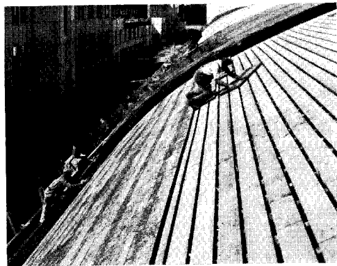
View showing placement of insulation serving as the bottom form of the arch.
