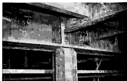
Hatch end beam supported by main pillar carries longitudinal stringers and girders, which in turn support deck beams.
