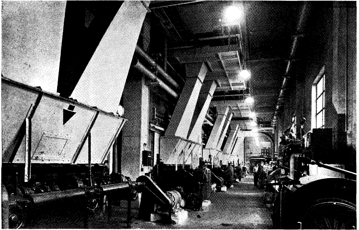
View of boiler room in separate building. Boilers are for heating only, as electric power is provided by the local utility company
