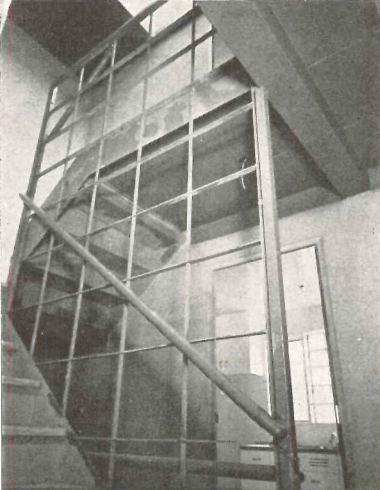
Fig. 8. Steel construction including box sections filled with concrete and used as ceilings. River Forest Garden Apartments, Chicago, Illinois, Holsman & Holsman and Klekamp, architects. The author proposes that this kind of steel ceiling form be so adapted that the concrete filling could be given credit for its inherent structural contribution
