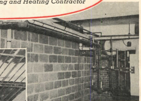
Heating and plumbing services—Hot and cold water lines, gas lines and waste and vents under 2-inches, are Byers Wrought Iron.
