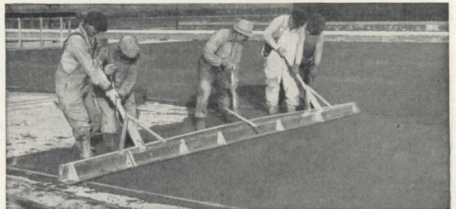
● Screeding Zonolite Insulating Concrete roof fill over concrete slab. Easily formed into saddles and cants for proper drainage.
