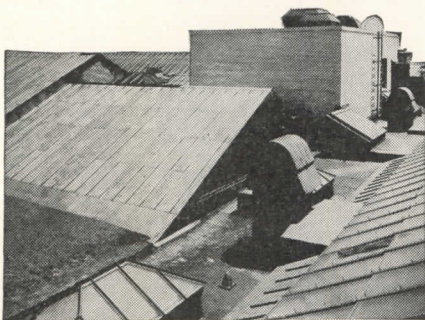
ON THE ROOF. Section of Monel standing seam roofing and Monel skylight caps and trim installed on The New York Historical Society by J. J. Fisher, Brooklyn, N. Y.
