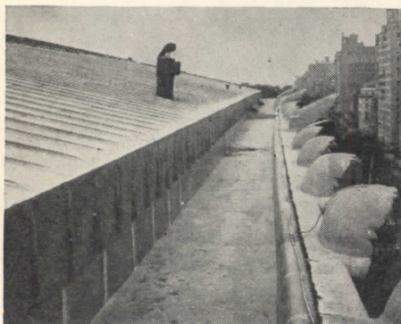
VIEW OF MONEL GUTTER and section of standing seam roofing and flashing installed in 1936.
