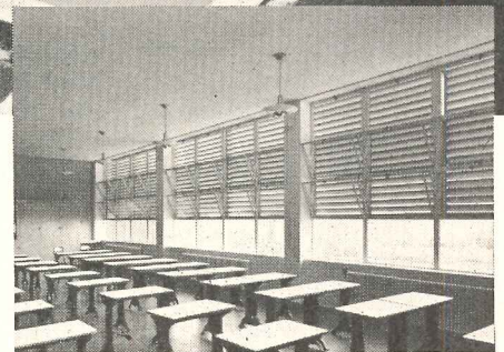
Stationary steel louvers were employed to control light, deflecting it to the ceiling.
