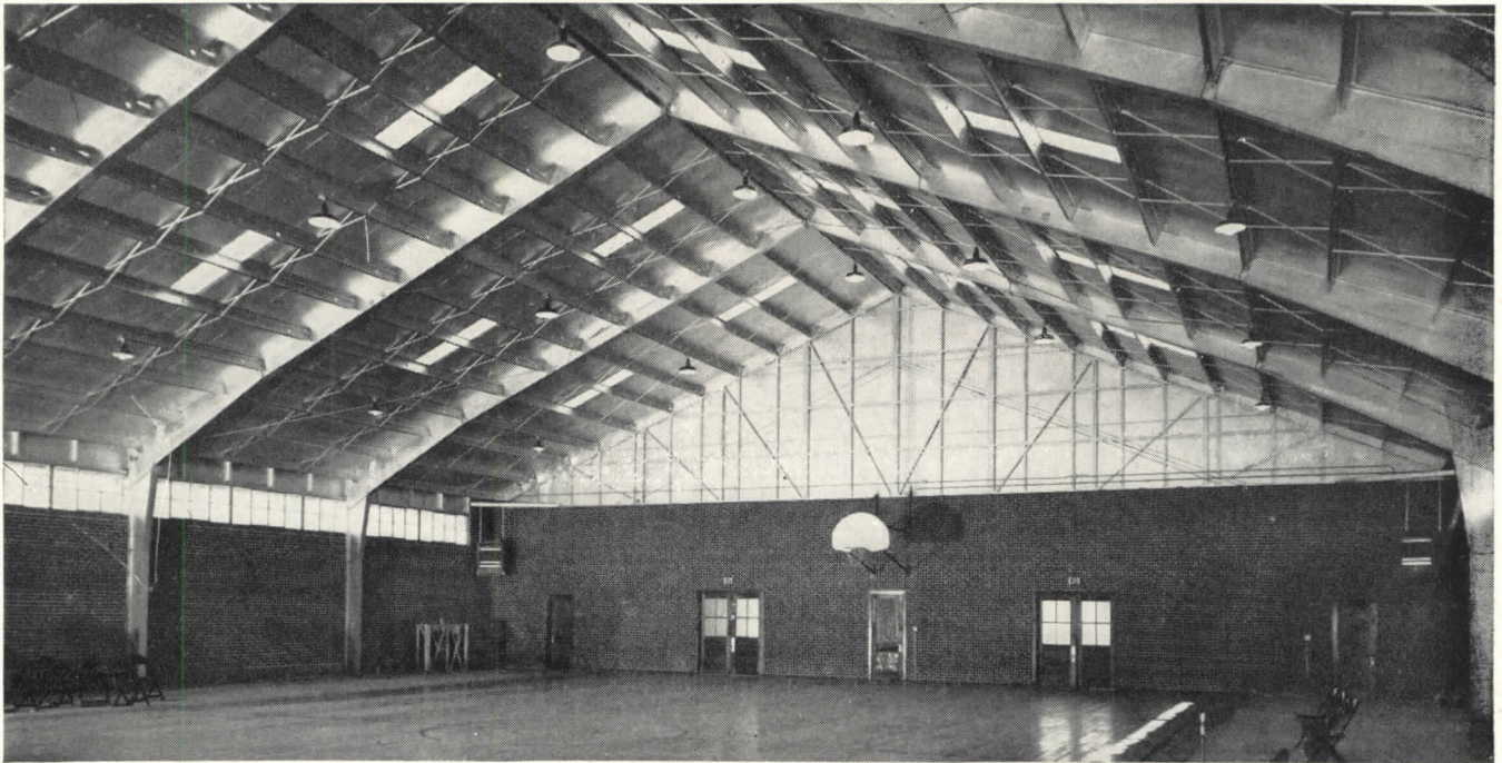
School gymnasium, 82' x 120', at Wright City, Oklahoma. Designed by David R. Graham, Tulsa, Oklahoma. Has clear, unobstructed view from everywhere. Note simple, compact roof construction.
