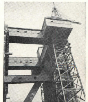
EXCELLENT CORROSION-RESISTANCE. Siding, roofing, gutters and leaders are Monel on the Sherman Creek coal hoist. The 37 years of service that this installation has seen have had little or no effect.
