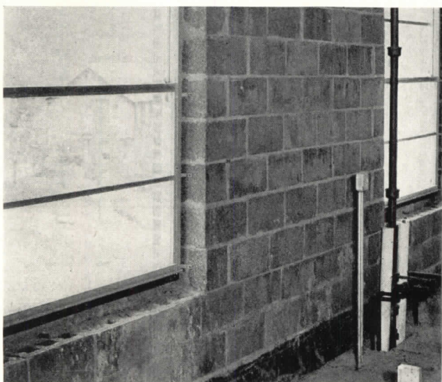
Above: concrete block backup fitted around window without any cutting. Below: interior tile wainscots also fit perfectly
