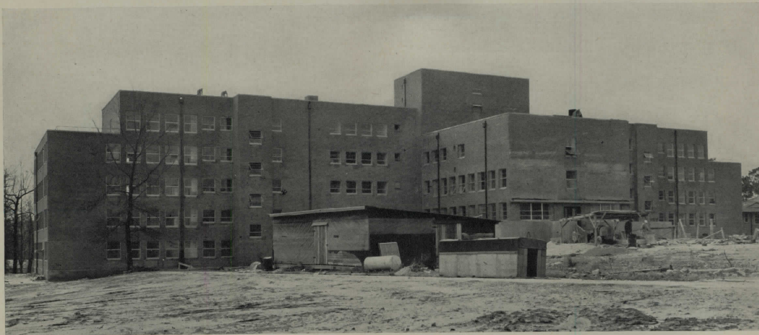
Mississippi adds 166 beds to its program for controlling tuberculosis among its negro population with this infirmary, shown here in construction views, an addition to an existing institution. Upper view shows principal facade, facing south
