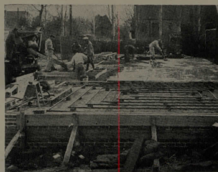
Today steel pipe coils are embedded in floors or ceilings during initial construction to provide advantages of radiant heating.
