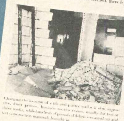
Changing the location of a tile and plaster wall is a slow, expensive work, while hundreds of pounds of tiles are carried out and wet concrete materials brought in.
