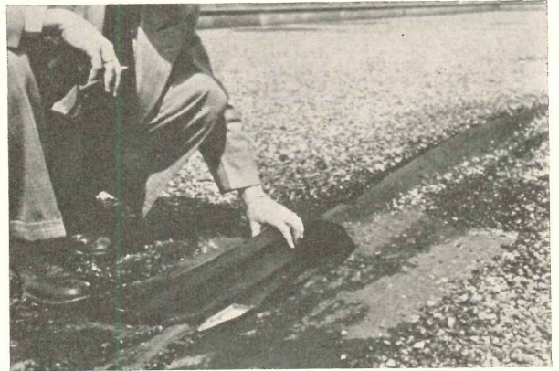
Expansion of air and water vapor stretches roofing, forms blisters
