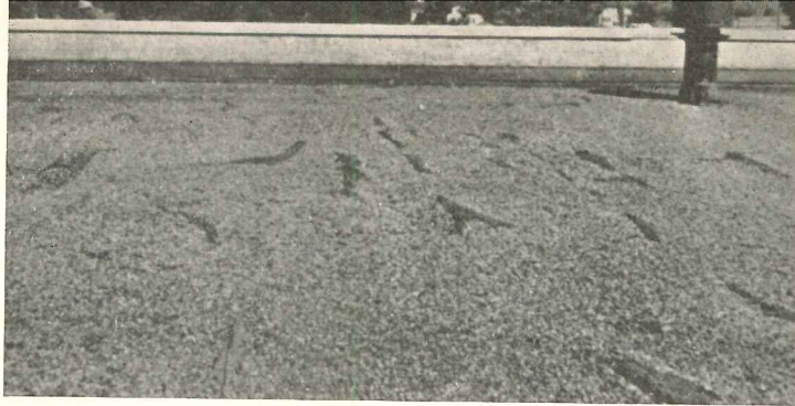
Continuous stretching, contraction of roofing results in "alligator" ridges
