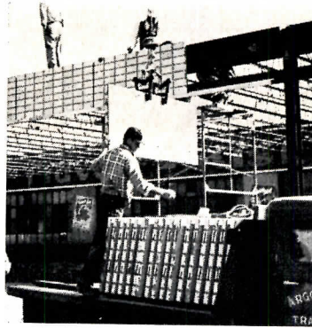
Pre-cast brick panels are stacked on truck and delivered to the job site
