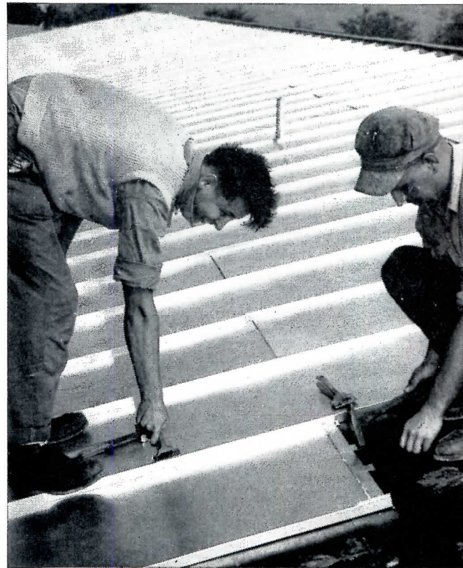
INSTALLING the standing-seam USS Stainless Steel roof on the new Walnut Grove School. The roof was laid on double-coated asbestos felt with each cross seam carefully caulked before the upper sheet was installed.
