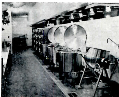
Closer view of kettles and steam cookers shows removable drains in stainless steel gutter and powerful furred-in exhaust hood above
