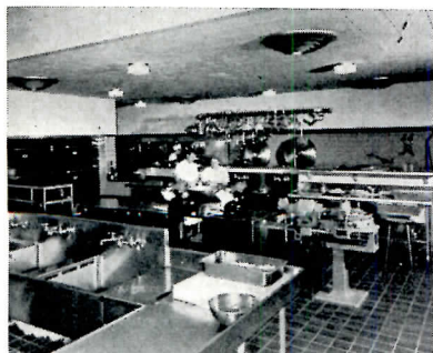
Vegetable and potato preparation area in South Quadrangle, University of Michigan. Kettles, steam cookers in background; ovens left. Air diffusers in ceiling
