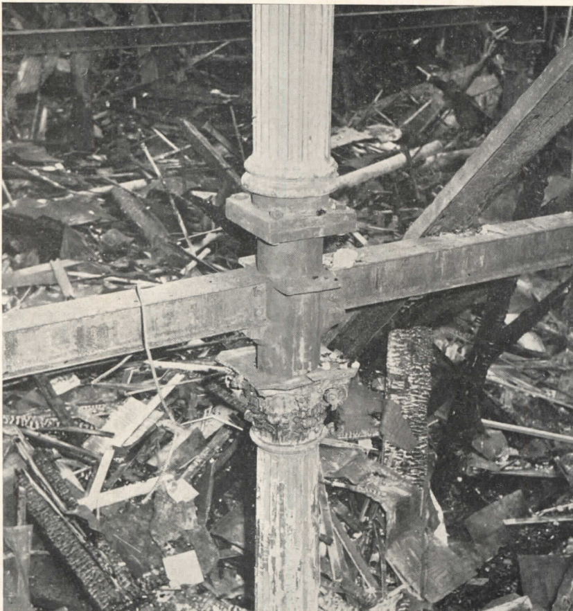
Detail of the column and beam connections. Beams rest on shoulder; appear to be two I-sections bolted through stub of casting
