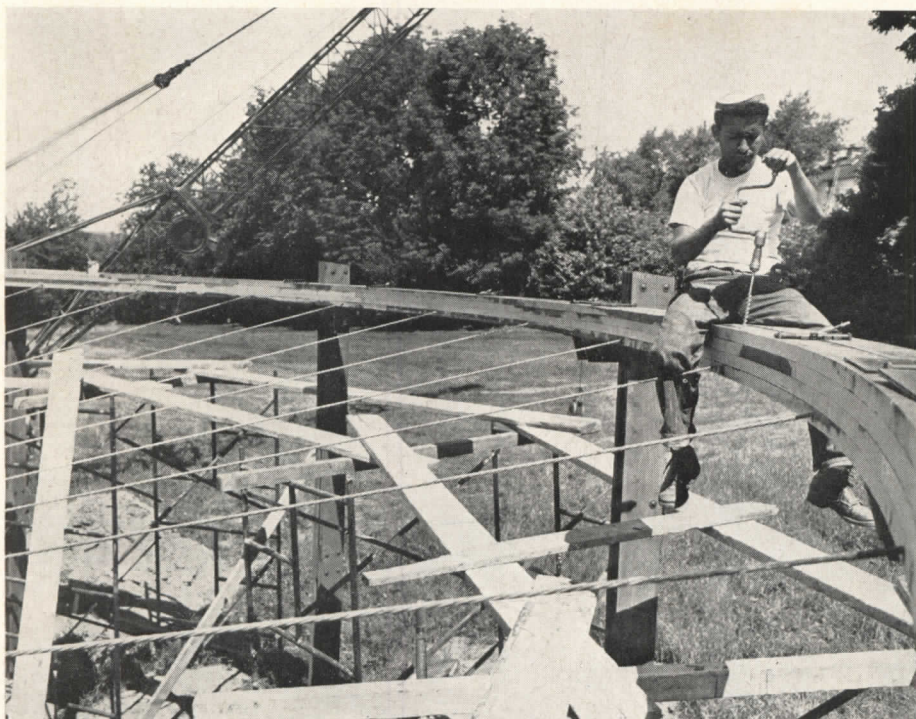
A laminated wooden ring holds steel cables at the circumference of Camp Columbia shelter
