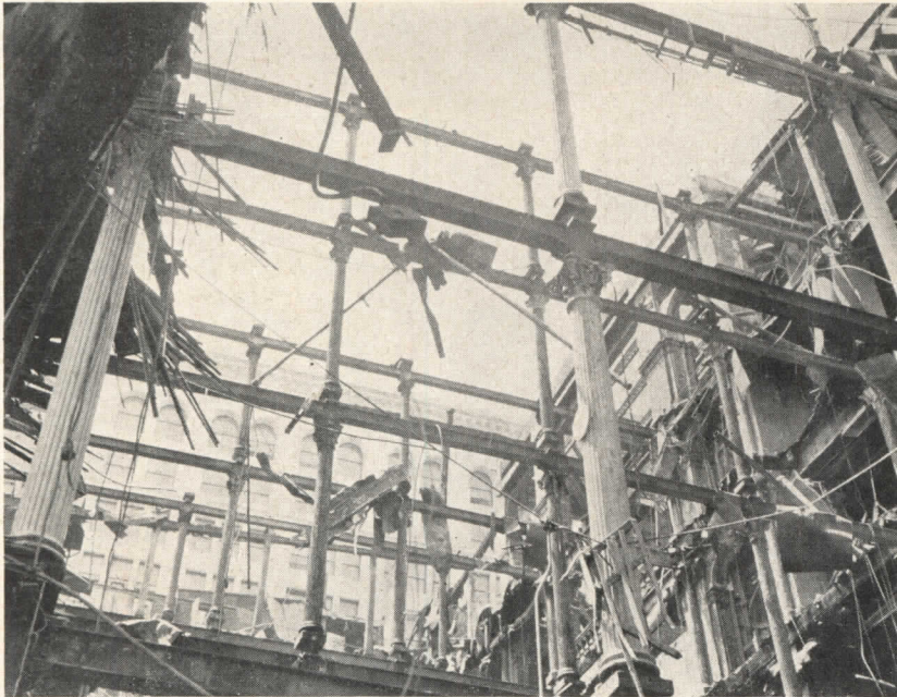
While fire has destroyed the wood joists, cast iron columns and wrought iron beams stand straight and true
