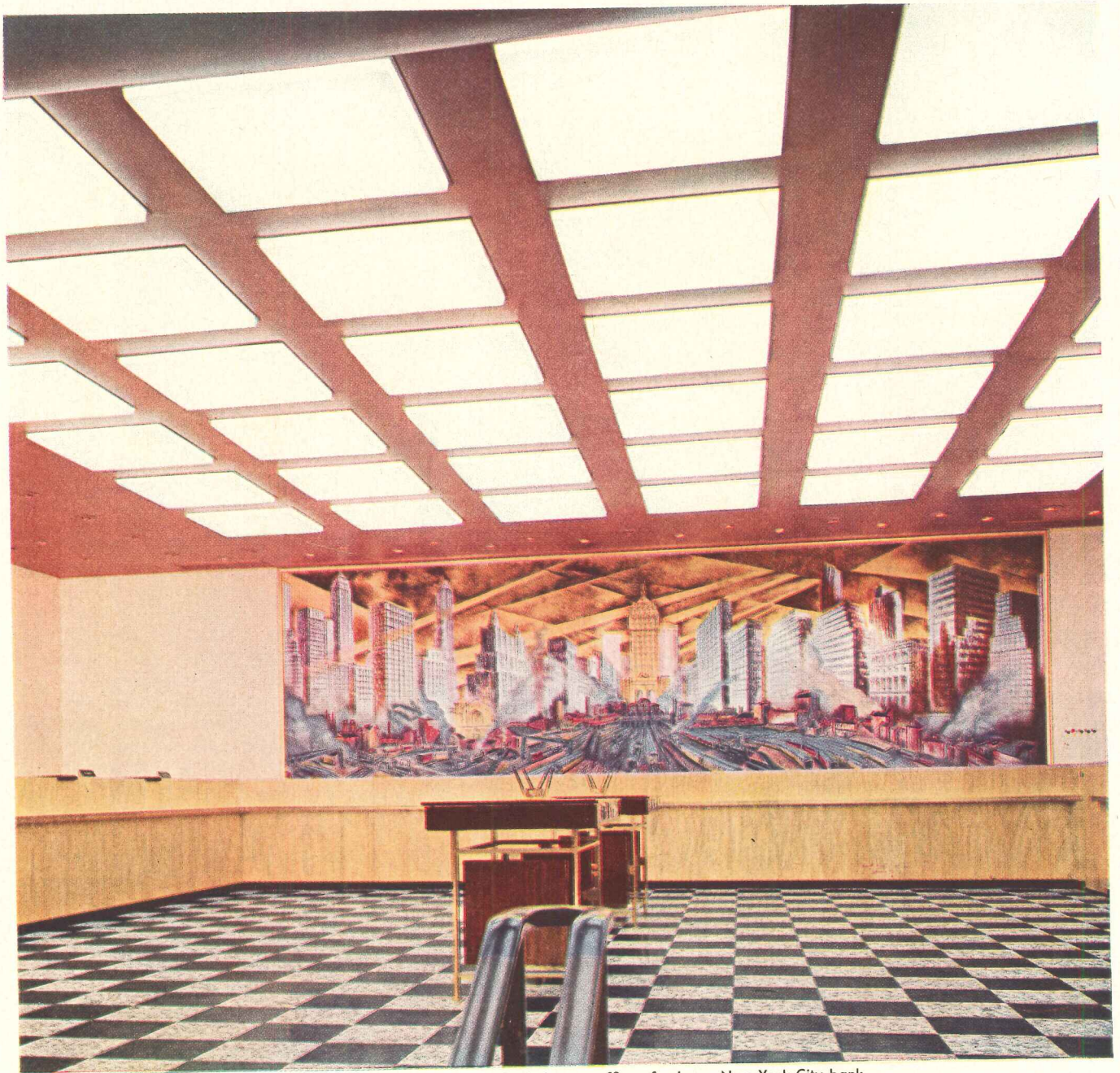
4'-square PLEXIGLAS diffusers at Park Avenue office of a large New York City bank
