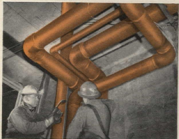
In the new Pittsburgh Hilton the hot, cold and chilled water supply is delivered by 130,000 lbs. of Types K and L Anaconda Copper Tube in sizes to 8".
