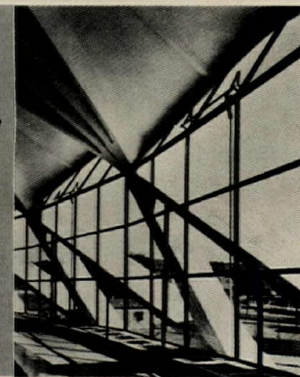
Detail of supporting arms. The Little Sports Palace, Rome. Annibale Vitellozzi , architect
