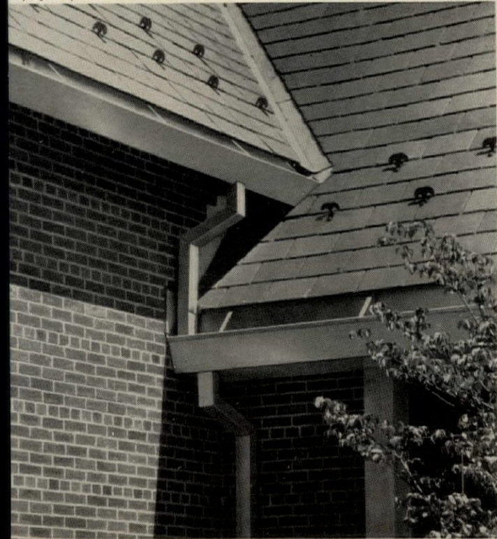
STAINLESS STEEL VALLEY FLASHING, valley flashing, gutters, downspouts, roof flashing and chimney flashing. Trinity Evangelical Lutheran Church, Latrobe, Pa. Architect: Mansell-McGettigan. General Contractor: Pevarnik Brothers. Roofing Contractor: Miller, Inc. and Gyekis, Inc.
