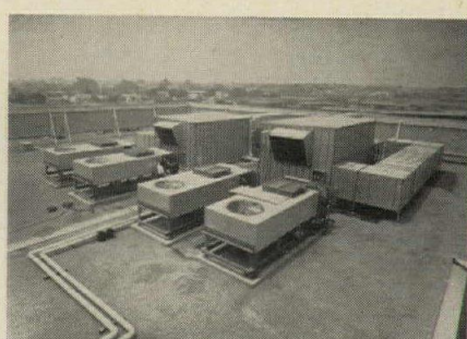
Easily accessible roof installed units.
