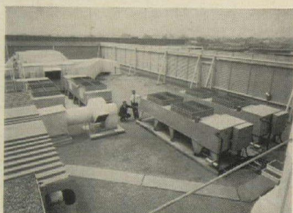
Roof top installation saves valuable space.
