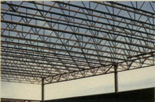
The open web feature of steel joists and joist girders allows ducts, pipes and wiring to pass directly through the steel members.
