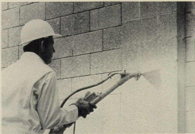
Spraying is the fastest way to apply BlocBond. Three men can cover about 1200 sq. ft. an hour.
