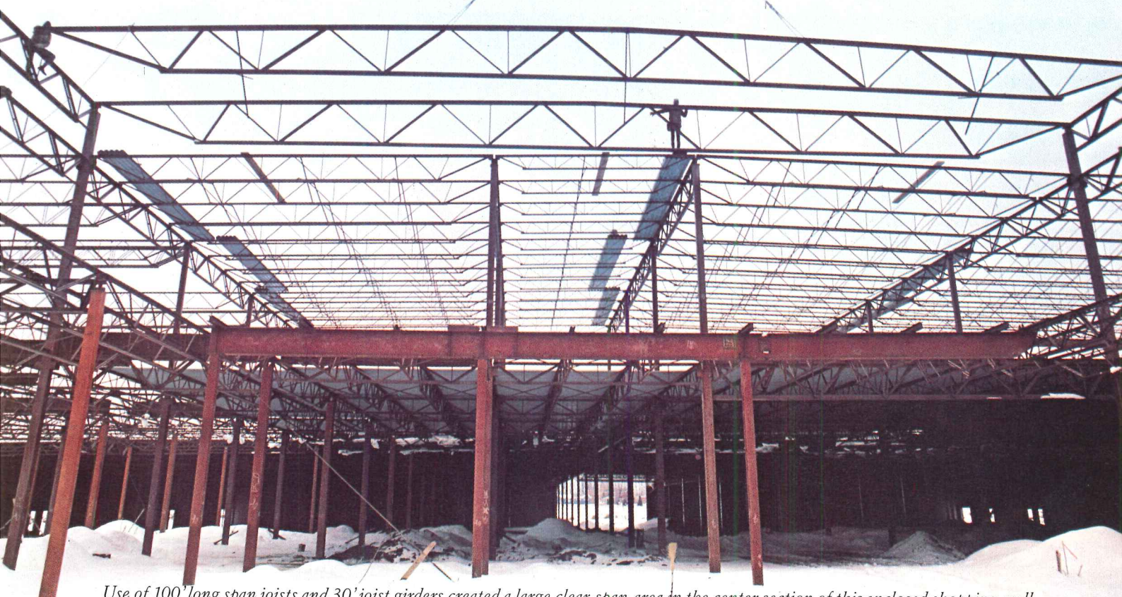
Use of 100' long span joists and 30' joist girders created a large clear span area in the center section of this enclosed shopping mall.
