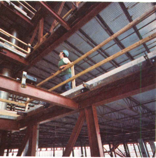
or view during construction shows large, column-free . Typical bays measure 53 ft 6 in. by 22 ft. Bethlehem ed 700 tons of structural steel for the project.
