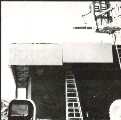
Educational Center Building, Hagerstown, Maryland Architect: NES, Campbell and Associates. Manufacturer: Cem-Fil Corporation, Nashville, Tenn.
