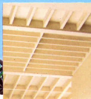
One-way joist floor system was used throughout. Eye pleasing ribs are in an alternating pattern perpendicular or parallel to the shear walls and spandrel beams.
