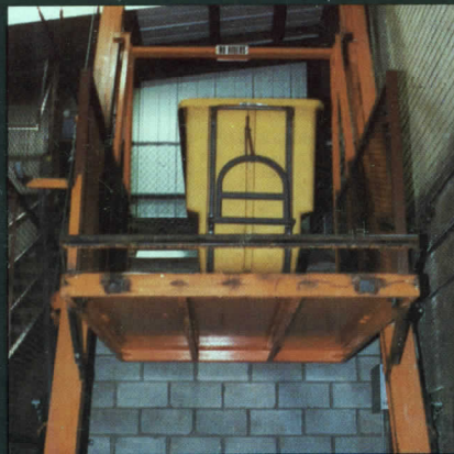
UCI 14: CONVEYING SYSTEMS
