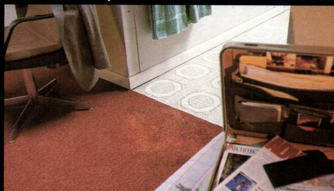
Damage and loss of color from harsh bleaches and cleaners.
