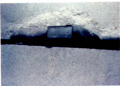
Ignoring stresses at clip angles, especially from movement of adjacent panels, can lead to spalling (above).
