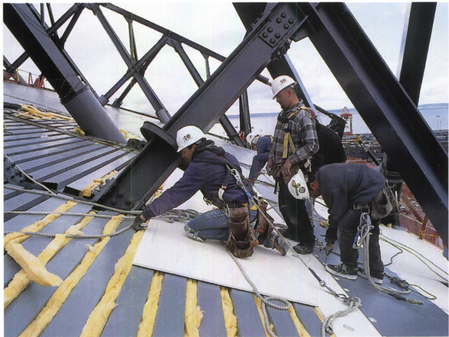
Working 200 feet in the air, roofers applied PVC to Safeco Field's roof.
