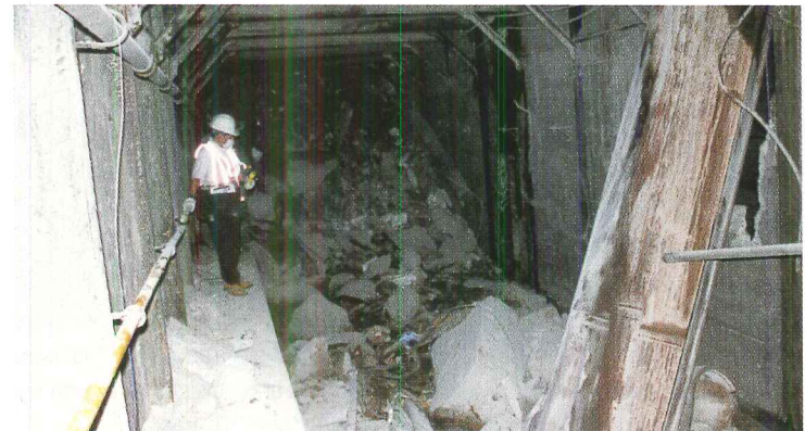
The 1/9 (top two) and N/R (above) subway tunnels incurred significant damage on September 11. Cost estimates to rebuild have not been announced.
