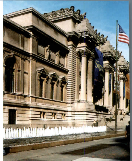
The Fifth Avenue facade of the Metropolitan Museum of Art, undergoing restoration by Wiss Janney, Elstner Associates.
