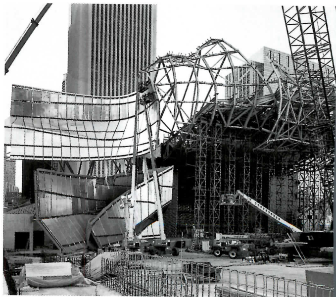
A view from afar of the park under construction (top); rendering of the Gustafson Garden (middle left); the Plensa
