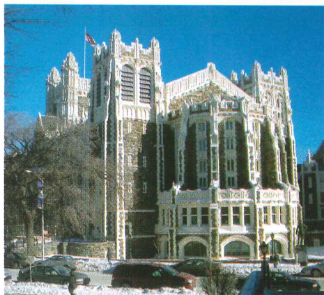
At Shepard Hall (above), masonry is replacing terra-cotta elements that were load bearing (top right). Before-and-after photos (middle and bottom right) show the new GFRC panels in action.
