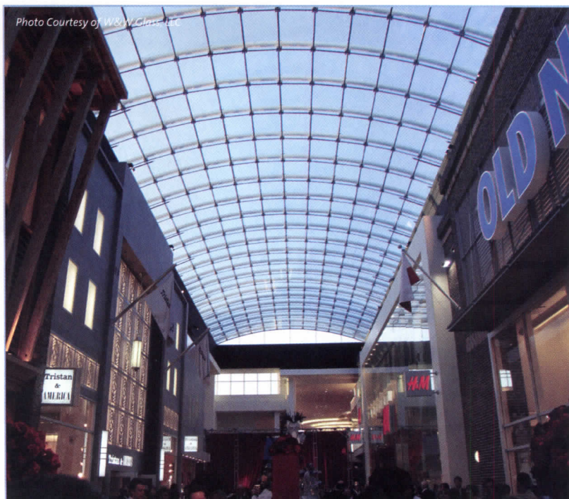
Transparency and performance are both enhanced with an ionoplast interlayer in the glass roof of Yorkdale Mall, Yorkdale, Ontario, Canada. Architect: MMM International Architects.
