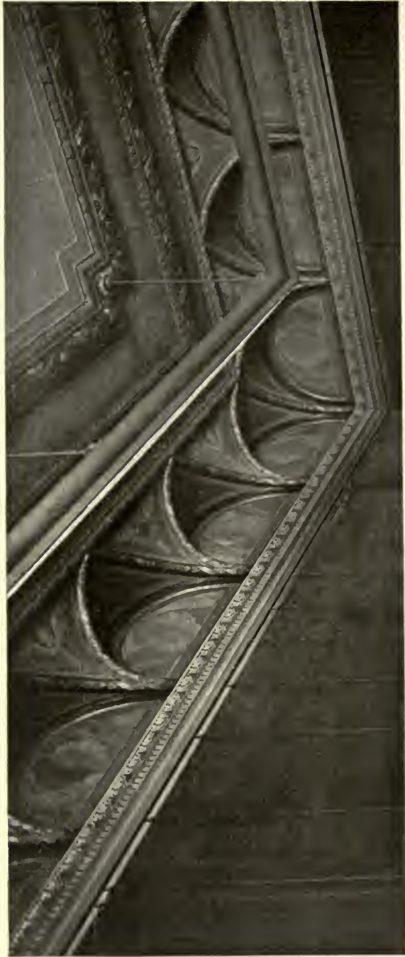
REAR GALLERY ON THE SECOND FLOOR— RESIDENCE OF COLONEL MICHAEL FRIEDSAM, NEW YORK CITY. FREDERICK G. FROST, ARCHITECT.
