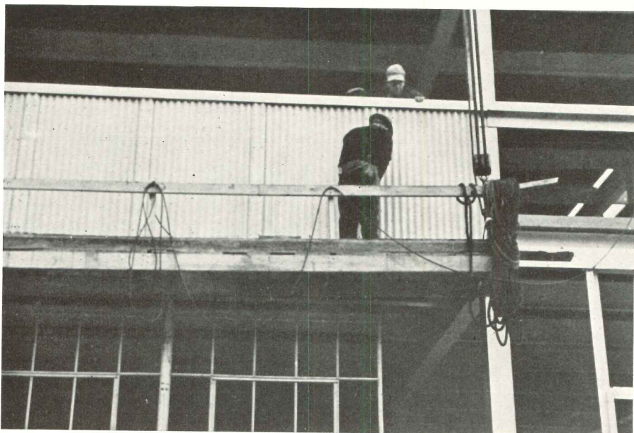
Large, lightweight rigid units make it possible for a small crew to erect many hundred square feet of curtain wall per day. The units come surfaced in either Flexboard (top) or corrugated Transite (below).
