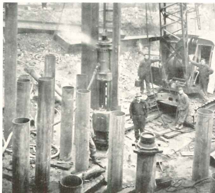
Even before being filled, this piling tested as high as 92 tons per pile.
