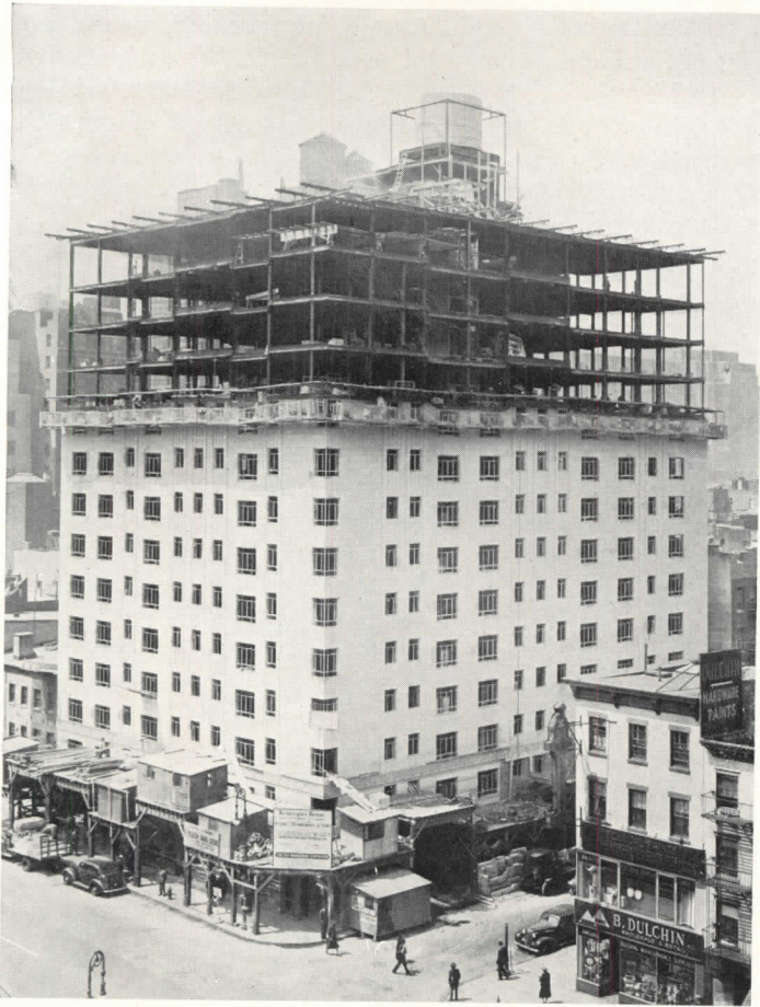
Fig. 15. A welded-frame apartment house recently completed in New York—first American city to amend its building code to permit welding.
