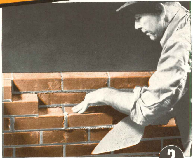
(1), it is much easier to shove the brick accurately into place, with a full head-joint, than it is to do the same thing with the other mortar (2).
