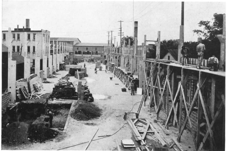
With the columns set in place, work can proceed quickly at all points
