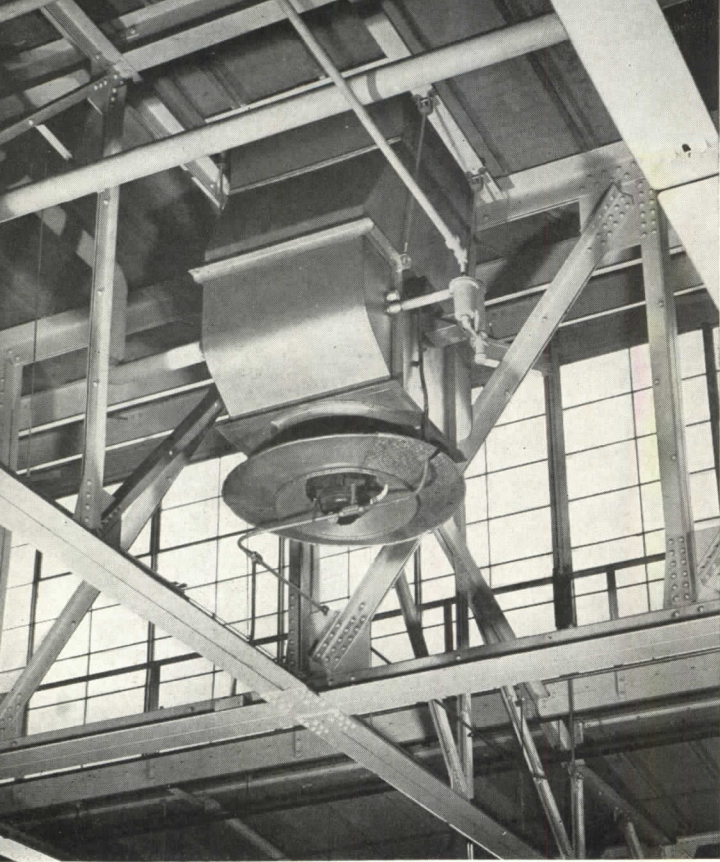
Another type of overhead unit heater used in the same plant. Unit heaters have the advantage that both steam and condensate return lines can be installed overhead through the trusses
