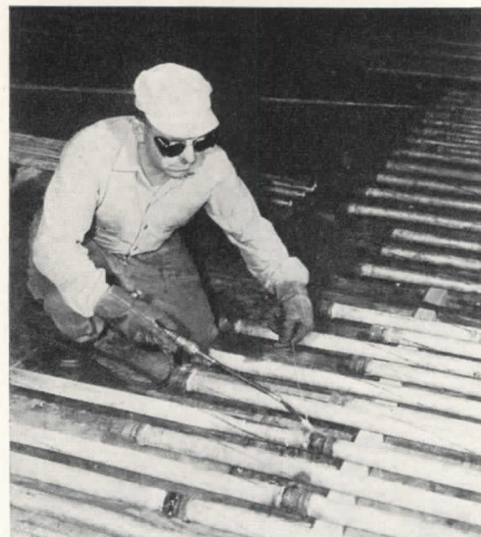
Operator applies silver alloy to braze threadless joint with piping in place
