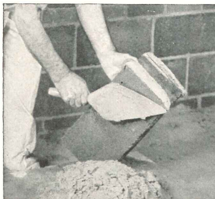
Method 1. Full head joints should be thrown onto both edges of the block to be placed, or—
