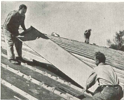
INSTALLING MONEL BATTEN PANS over wooden batten bars. The pans have pre-formed ends that provide watertight joints without solder. Monel nails and cleats are used to lock the pans and the Monel batten caps together.
