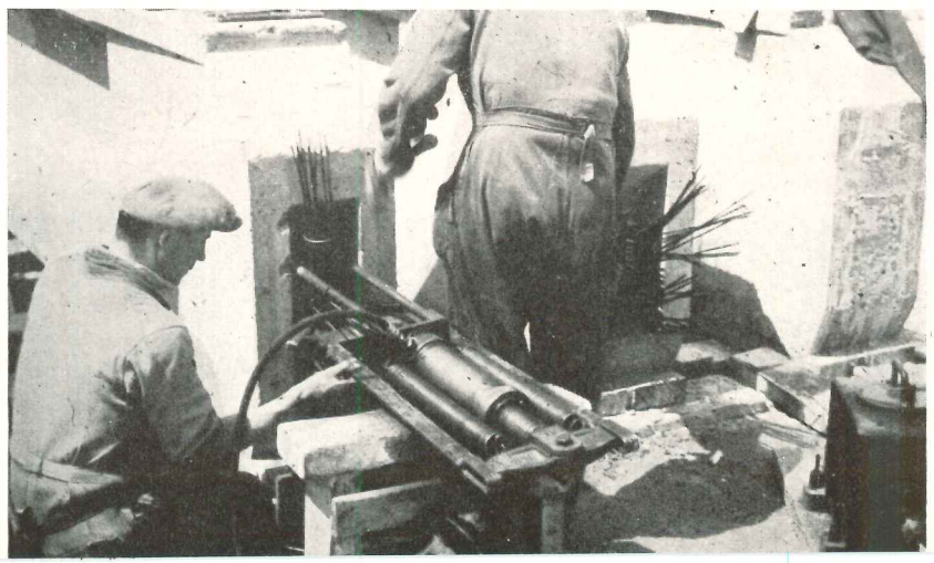
12, 13, 14, 15. Prestressing as done by the Belgian method. 12. End of girder before it is prestressed; cables are strung through beam after concrete is hard. 13. End of girder after wires have been tensioned by a hydraulic jack (14) and anchored by means of sandwich plates; pipes sticking out are for injecting grout after girder is prestressed
