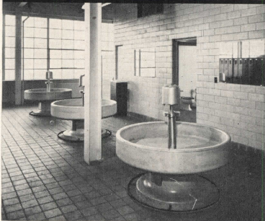
8 to 10 persons wash simultaneously at a Bradley 54-inch Washfountain.
