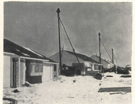
Plastic pipe is used to save cost in well installations for housing project
