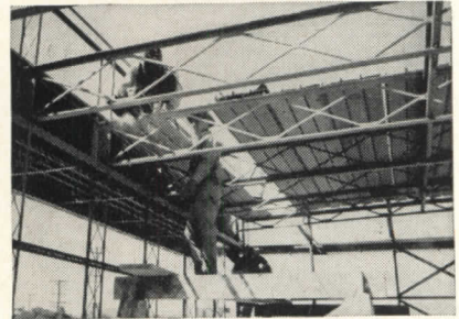
30% Less Steel required for this garden shop, built with welded design for Sears Roebuck & Company, Compton, California. Construction cost cut from $30,000 to $20,000.
