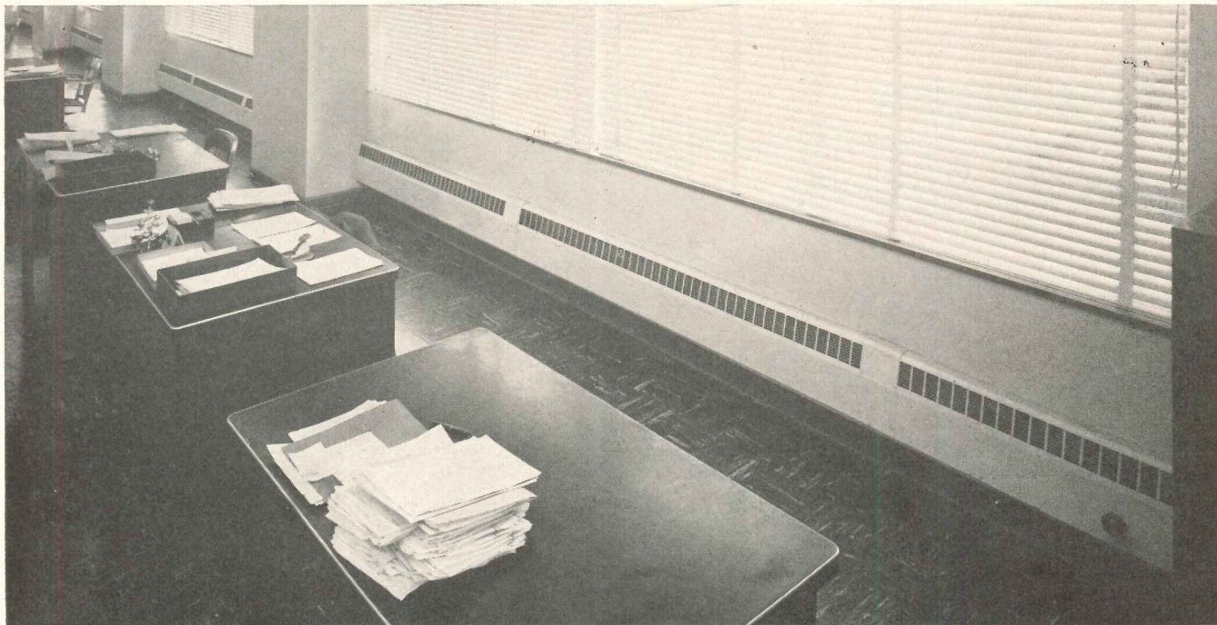
Typical view showing Webster Walvector ® providing heat the full window length, column to column. The steam risers and the returns are in alternate columns. Webster Radiator Valves provide shut-off of the heat in each bay.
