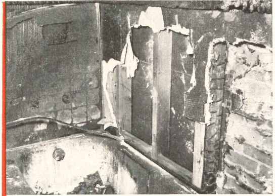
Right foreground shows section where firemen broke through FIRESTOP during blaze. Charred side of wooden stud is the result. Then compare remaining undamaged studs between the FIRESTOP wallboards. Wallboards were broken away after fire to show undamaged condition.
