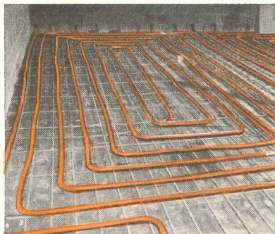
HEAT USED - Shown here is part of the 500 feet of copper coil embedded in concrete slabs in the floor of adjacent plant offices and other areas. This tubing circulates the refrigerant gas to furnish radiant heat.
