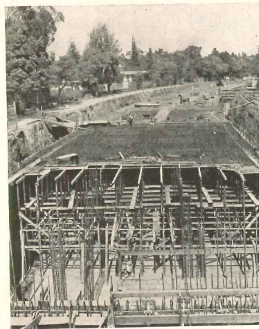
Above: the problem in a California reservoir was to gain watertight concrete under difficult placing conditions. A retarder and a workability agent were the admixtures. Below: concrete for this 4,750,000 gal. water tank had a cement-dispersing, water-reducing agent in it
